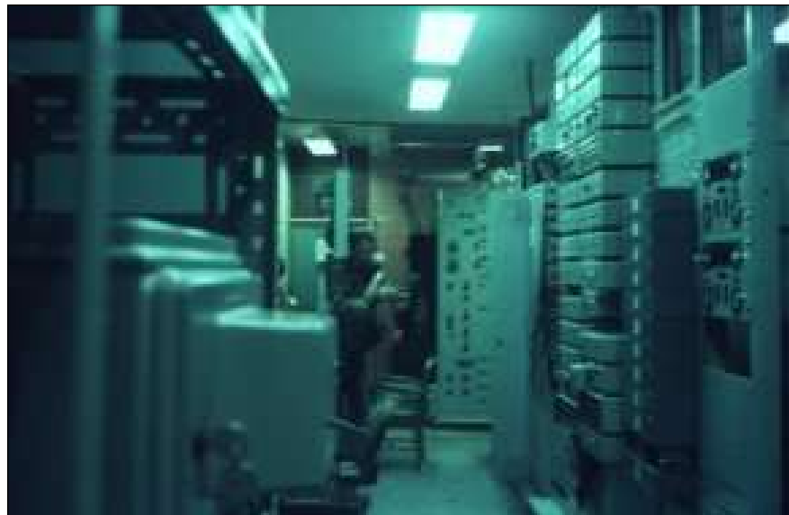
Photo 8.2 - Communication equipment at 110 Signal Squadron, Vung Tau (1970).
